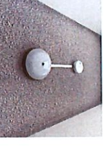
20. Lounge room - Fans/light fittings 21/05/26 at 10:09 AM
