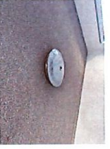
19. Lounge room - Fans/light fittings 21/05/26 at 10:09 AM
