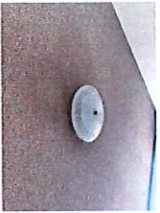
18. Lounge room - Fans/light fittings 21/05/26 at 10:09 AM
