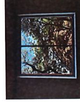
12. Lounge room - Windows/screens 21/05/26 at 10:06 AM
